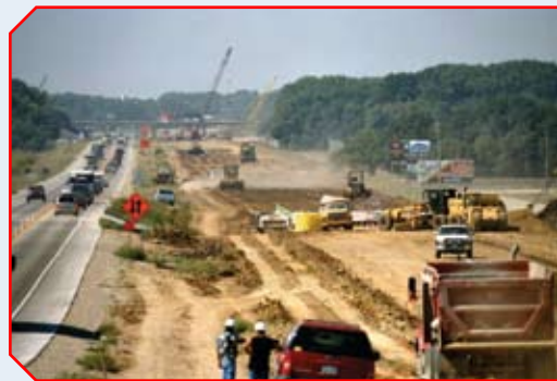
Near Salina, KS, I-70 is completely rebuilt under traffic. Photo courtesy Kansas DOT
